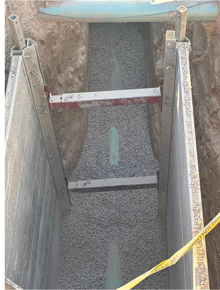
8" sewer main bedded in gravel
