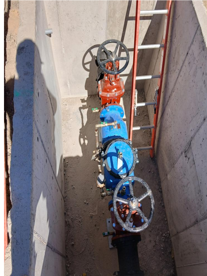
Inside DCDA vault
