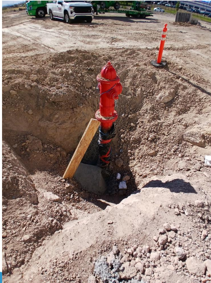
Fire hydrant with thrust block
