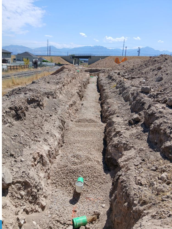
6" sewer lateral for rv dump
