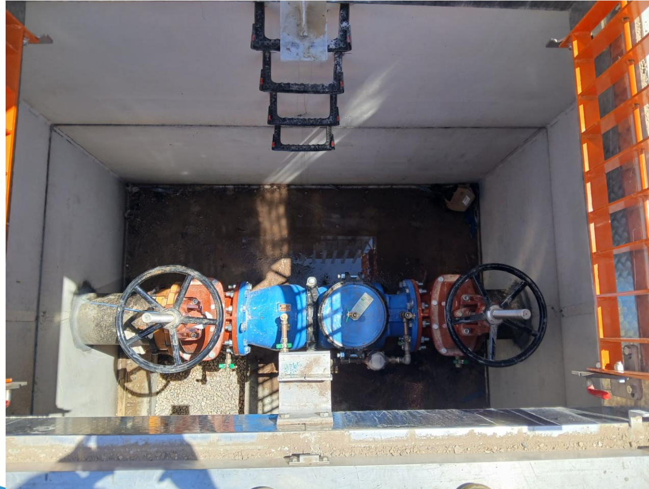
10" DCDA on fire line
