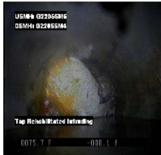
Figure 9: Depicts a lateral liner that was over shot into our main. The company responsible is coming to cut it out.
