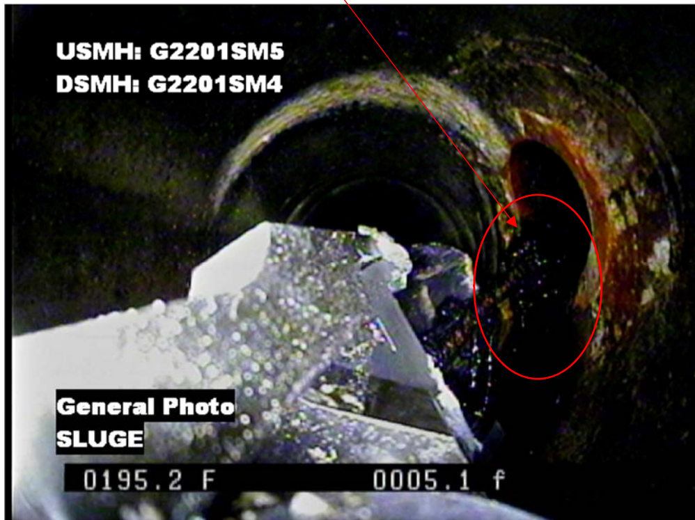
Figure 11: Depicts black sludge pouring into the sewer main as the lateral is being inspected.
