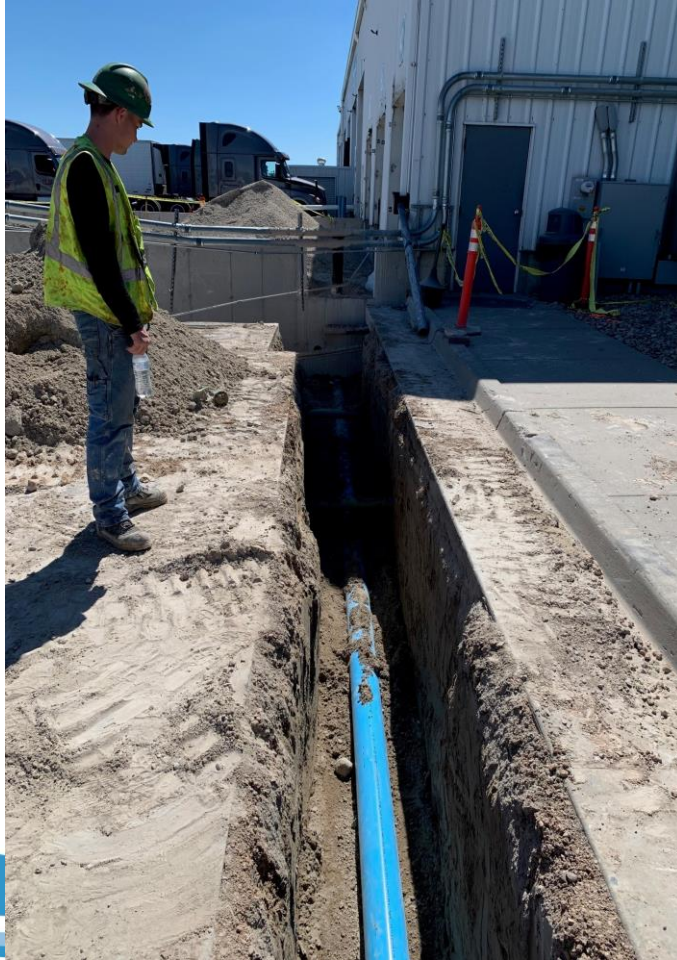
6" fire line entering building on north side
