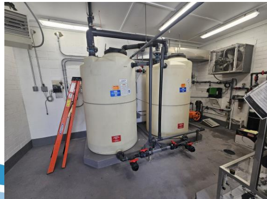
New fluoride tank installation
