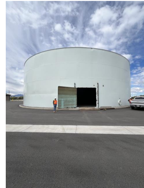
New fluoride tank installation
