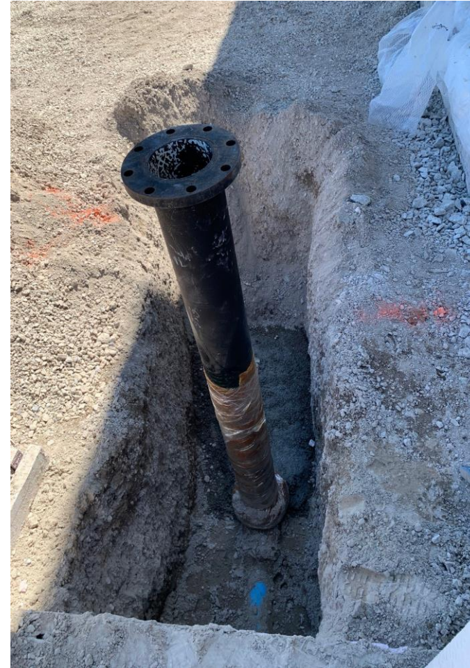
6" riser with thrust block inside building
