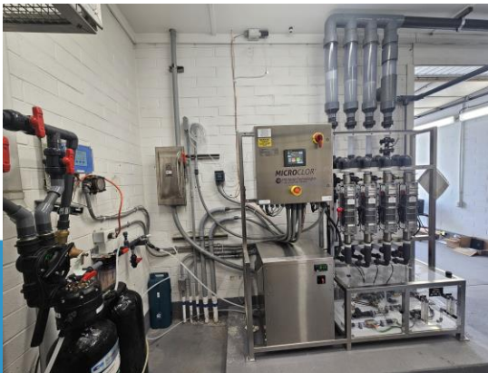
New PSI Sodium Hypochlorite system
