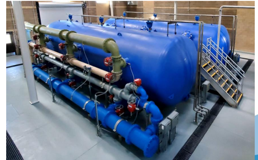
Rushton WTP filter vessels
