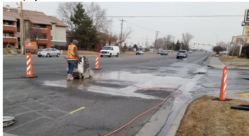
Redwood Road Main Break
