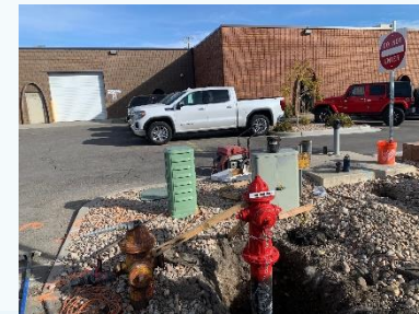
New fire hydrant
