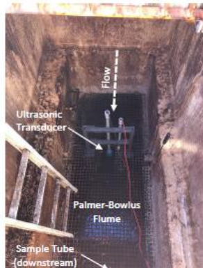
Example Flow Metering Structure (Murray City)
