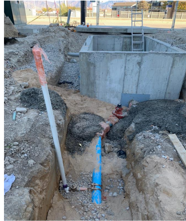
Valve, pipe, and fittings behind vault on customer's side
