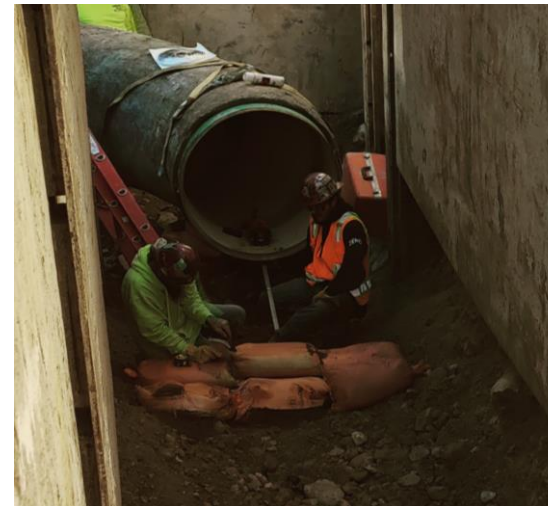
Workers in deep trench (with shoring) setting up sandbags to provide support underneath 36" welded steel pipe
