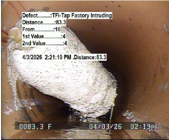
Intruding lateral liner @ 4480 S 3600 W (Culprit of SSO)
