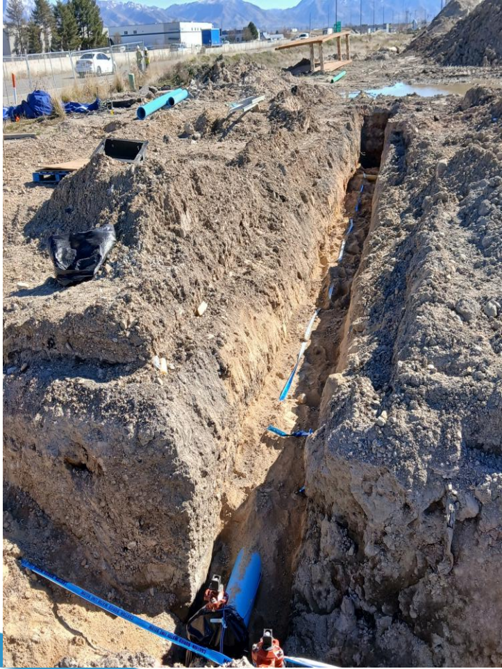
8" fire line stubbed into property
