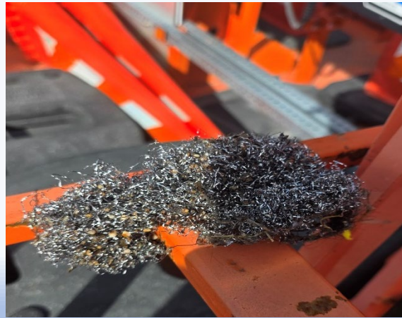
Metal Shavings removed from main line. Which have been causing havoc at CVWRF.
