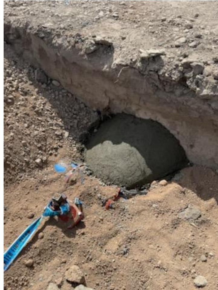
Thrust block behind fire hydrant tee
