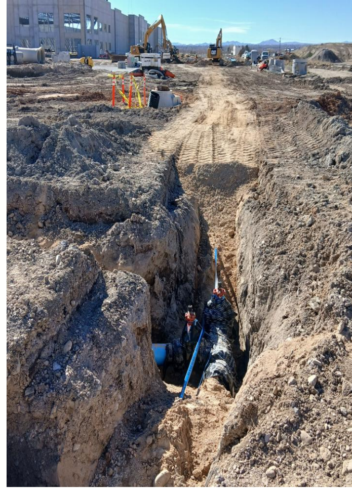
10" water line and valves
