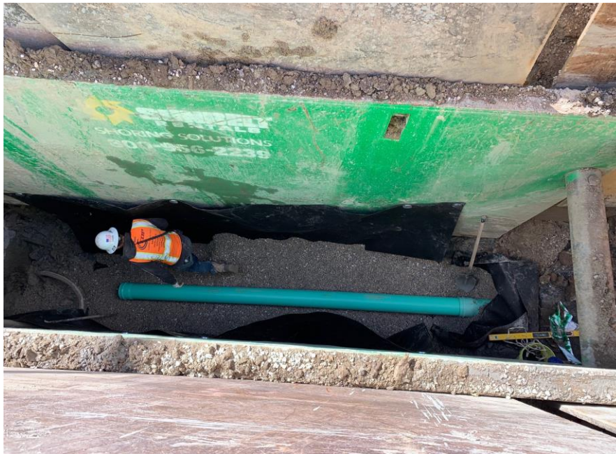
Typical sewer pipe installation - pipe on gravel bedding. Geotextile fabric held up with magnets on trench box walls.
