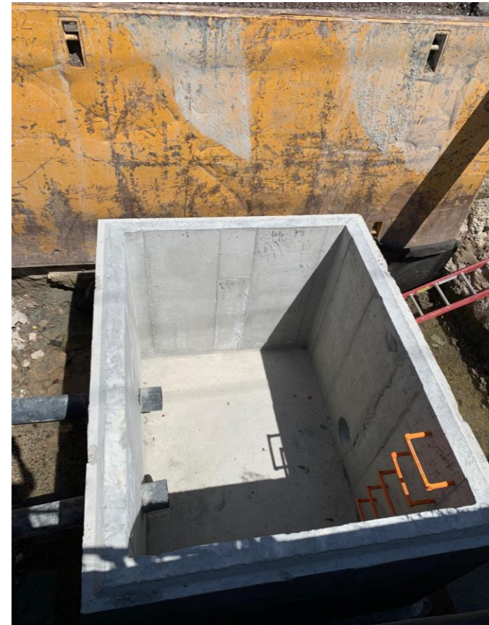
Pig retrieval vault with two 8-inch force mains.
