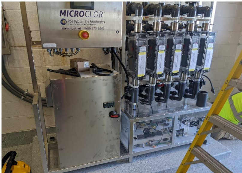
Well No. 15 Chlorinator Installation
