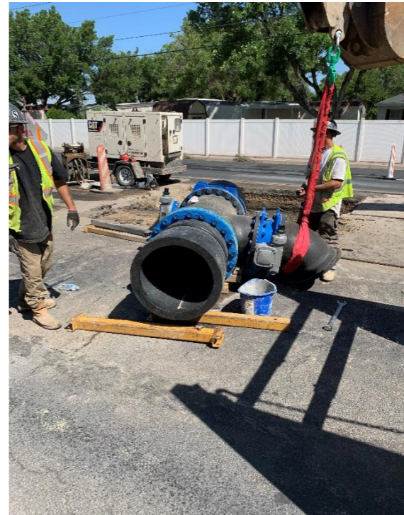
28-inch HDPE Tee
