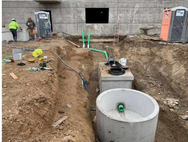
Grease interceptor and sampling manhole
