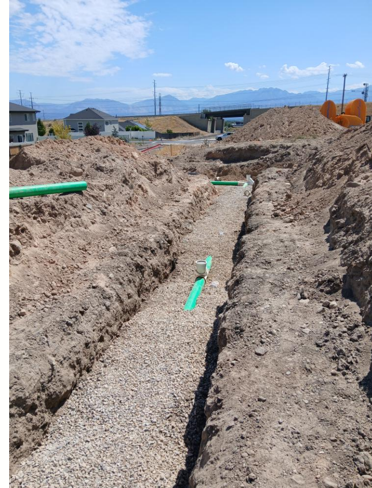
6" sewer lateral with cleanouts
