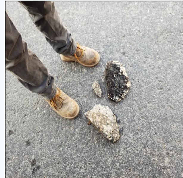
Depicts large chunks of concrete that were found in our sewer main, due to the contractor not placing boards in the manhole while being lowered and having new concrete aprons poured.
