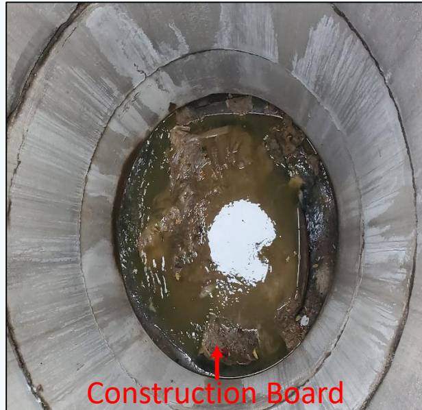
This image depicts a construction board beginning to plug off the sewer main on 4100 S and Blue Jay St.
