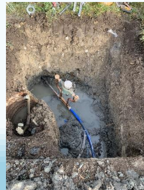
New meter assembly connection
