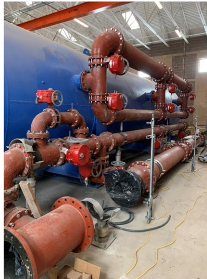
Filter vessel piping
